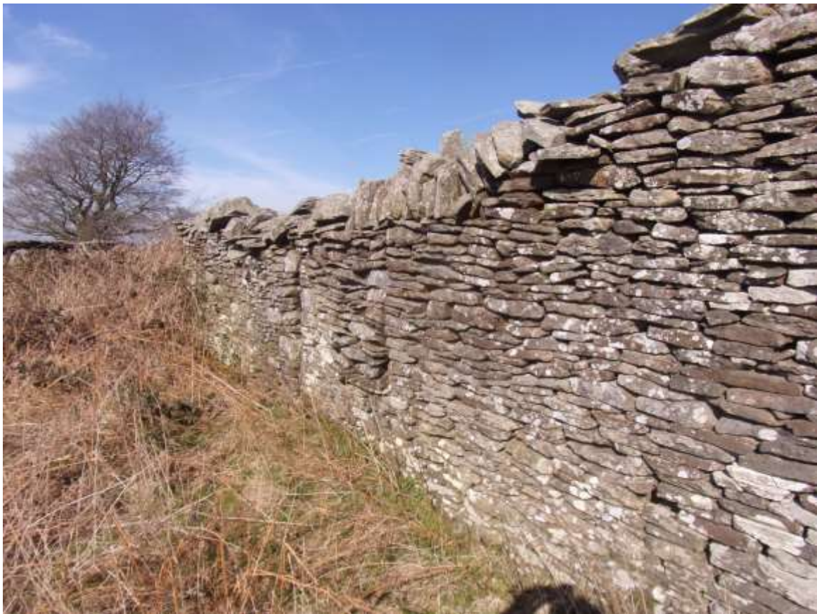
Figure 6 The front of Ty Shors showing fine dry stone construction and rubble filled window space. (RJS)
